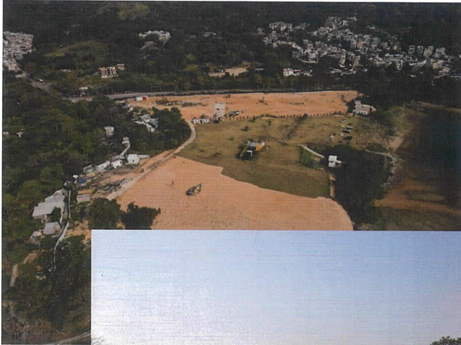
Figure 3-4 During our current site visit in early January 2025, site formation work in large scale is taken place. Signs of vegetation clearance and tree felling can be observed
